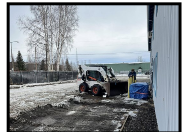
Above photos: Plowing the water and snow away from the building, 4/5/25, to prevent office flooding.
