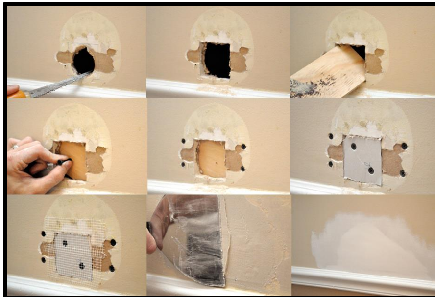
Figure 1: Sheetrock hole repair. Ethan. 1 June 2018. One Project Closer, How to Repair a Medium-Size Hole in Drywall, https://www.oneprojectcloser.com/how-to-repair-medium-size-hole-in-drywall/ .
